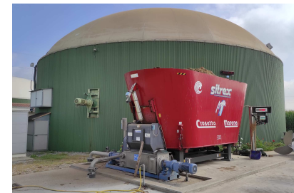
Screw charger and digester
