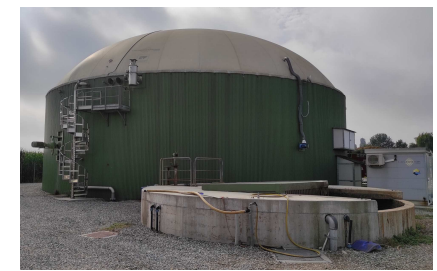
Inlet tank and digester
